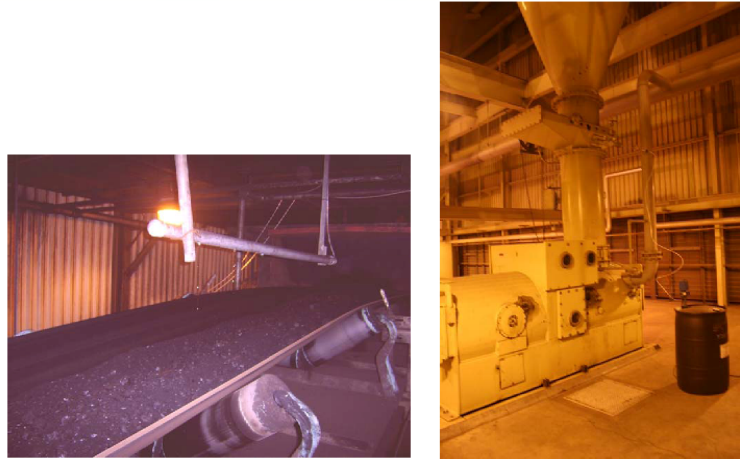
Figure 3. Typical KNX Addition Locations: Coal Belt (L); Coal Feeder (R)
